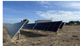
Palmeri PV Plant 1 MW
