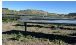
SAV PV Plant 1 MW
