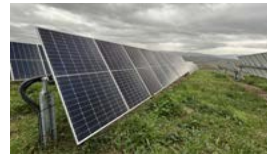
Favari PV Plant 1 MW
