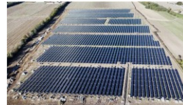
Rivarolo PV Plant 11 MW
