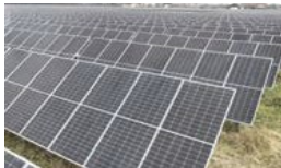
Indovina PV Plant 1 MW
